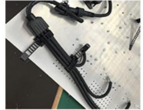
Solar controller wiring
